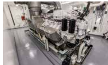
Wärtsilä 14 auxiliary generator.
