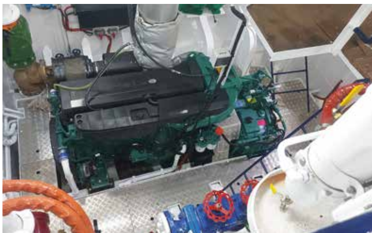
Volvo main engine and gearbox.
